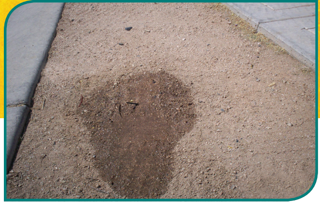
It is important to plug all unused emitters even though the water loss is insignificant compared to water used to irrigate turf areas.
