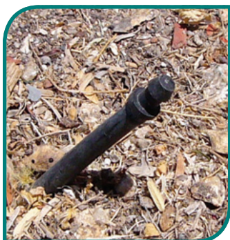
A drip tube that has been capped.
